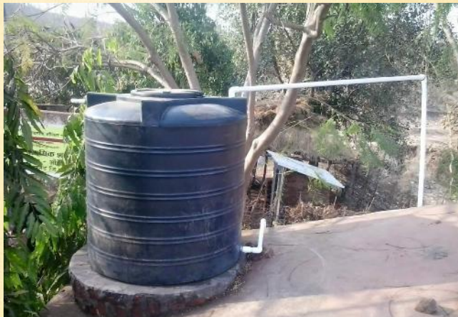
Overhead water tank for water storage
